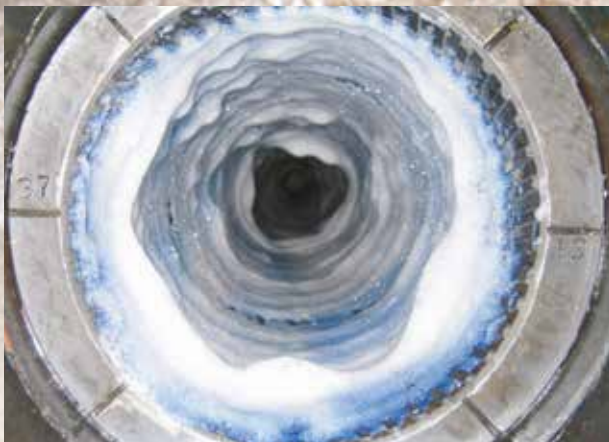
Foam discolouring in blue. Evidence of copper.
